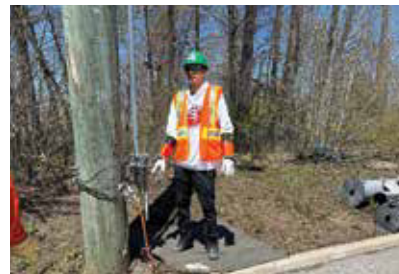
Jarrett Mark learning how to safety turn Off and On "3 Phase Overhead Switch"
